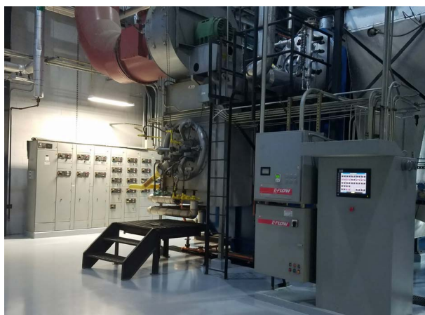
The steam plant is located at the base of the bell tower and is the single largest Scope 1 emissions source on campus.
