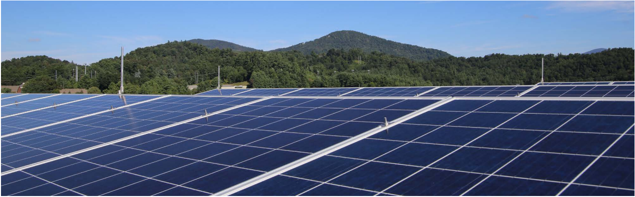
The PV system on the roof of Leon Levine Hall is comprised of 214 panels, with 57.8kW of capacity.
