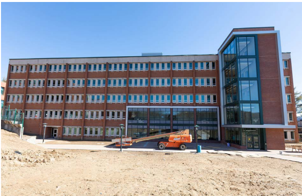
Reducing energy consumption in state-owned buildings is a goal of NC Executive Order 80. Among the renovations made to Sanford Hall are 464 energy-efficient replacement windows.
